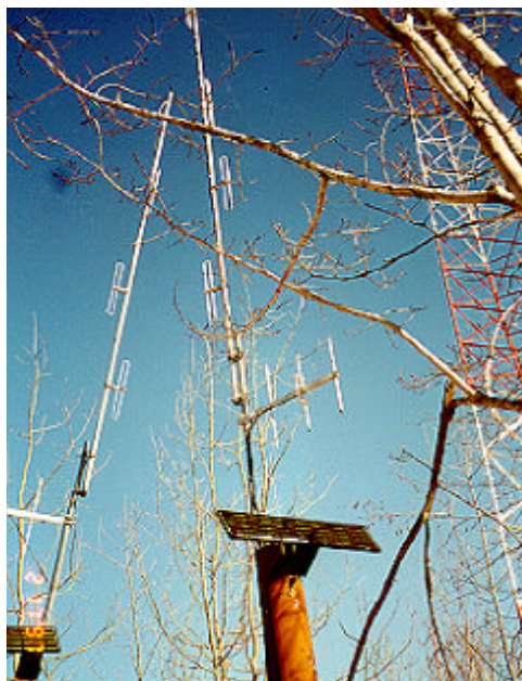
Solar Powered @ BCPD Tower
